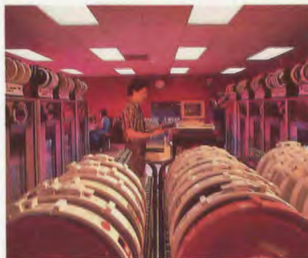
High-speed data capability serves the communications needs of large EDP centers.
